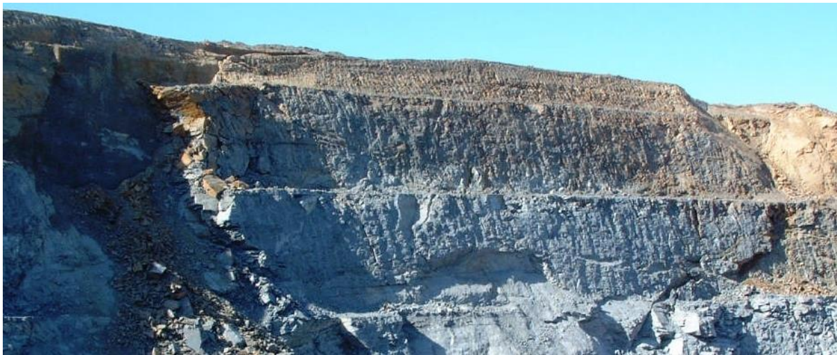
Figure 1. Photograph of pit area involved with slope failure.
